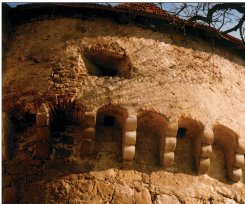
Fig. 43 Veliki Tabor castle: superstructure supported by corbels around the whole fort (photo by: Z. Horvat)
