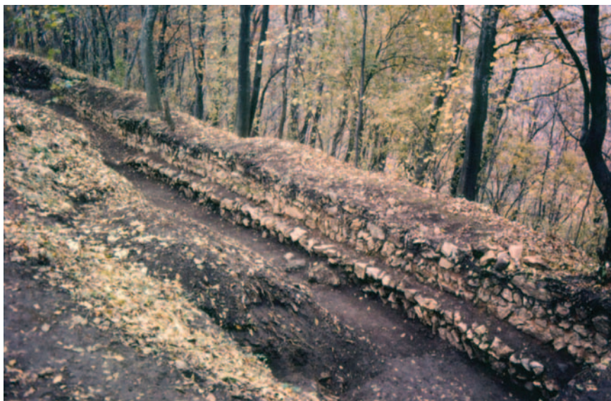
Fig. 1 Inner side of the Roman defensive wall – east (photo by: V. Sokol)
