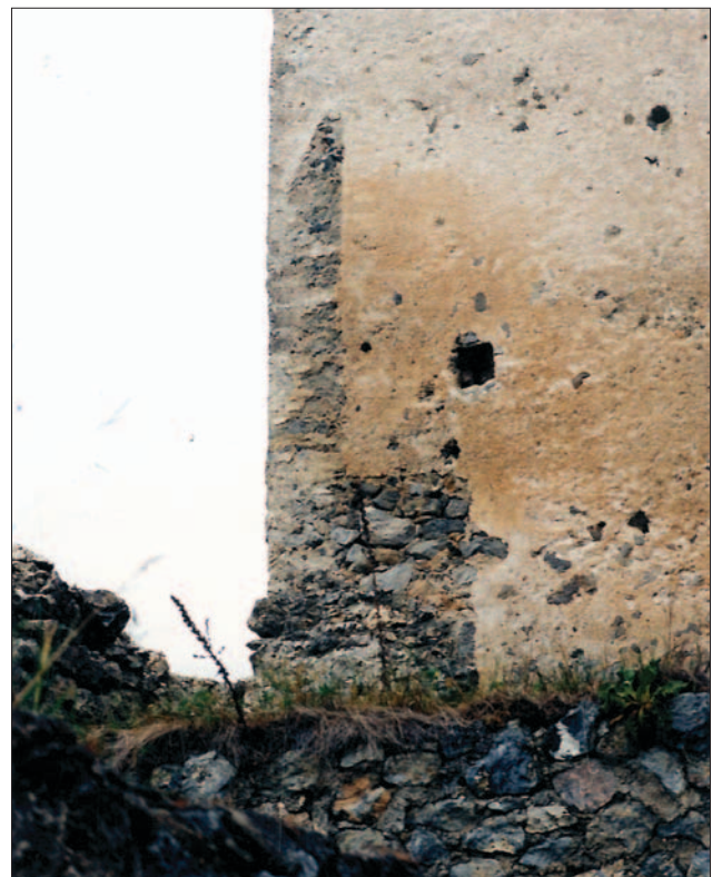
Fig. 10 Ružica castle, the second half of the 15 th century: 'negative' of a crenellation's cross-section visible on the so-called Renaissance palas (hall) (photo by: Z. Horvat)
