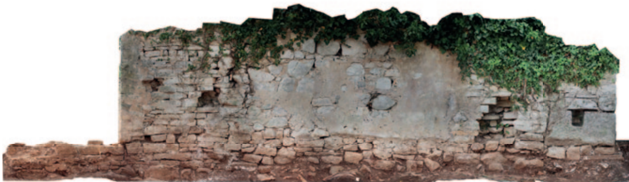
Fig. 2 Orthophoto of the rear wall of the Church of the Holy Cross and a segment of the earlier wall (photo and processing by: K. Bartolić Sirotić) Sl. 2 Ortofoto snimak začelja crkve sv. Križa i segment ranije arhitekture (snimila i obradila: K. Bartolić Sirotić)
