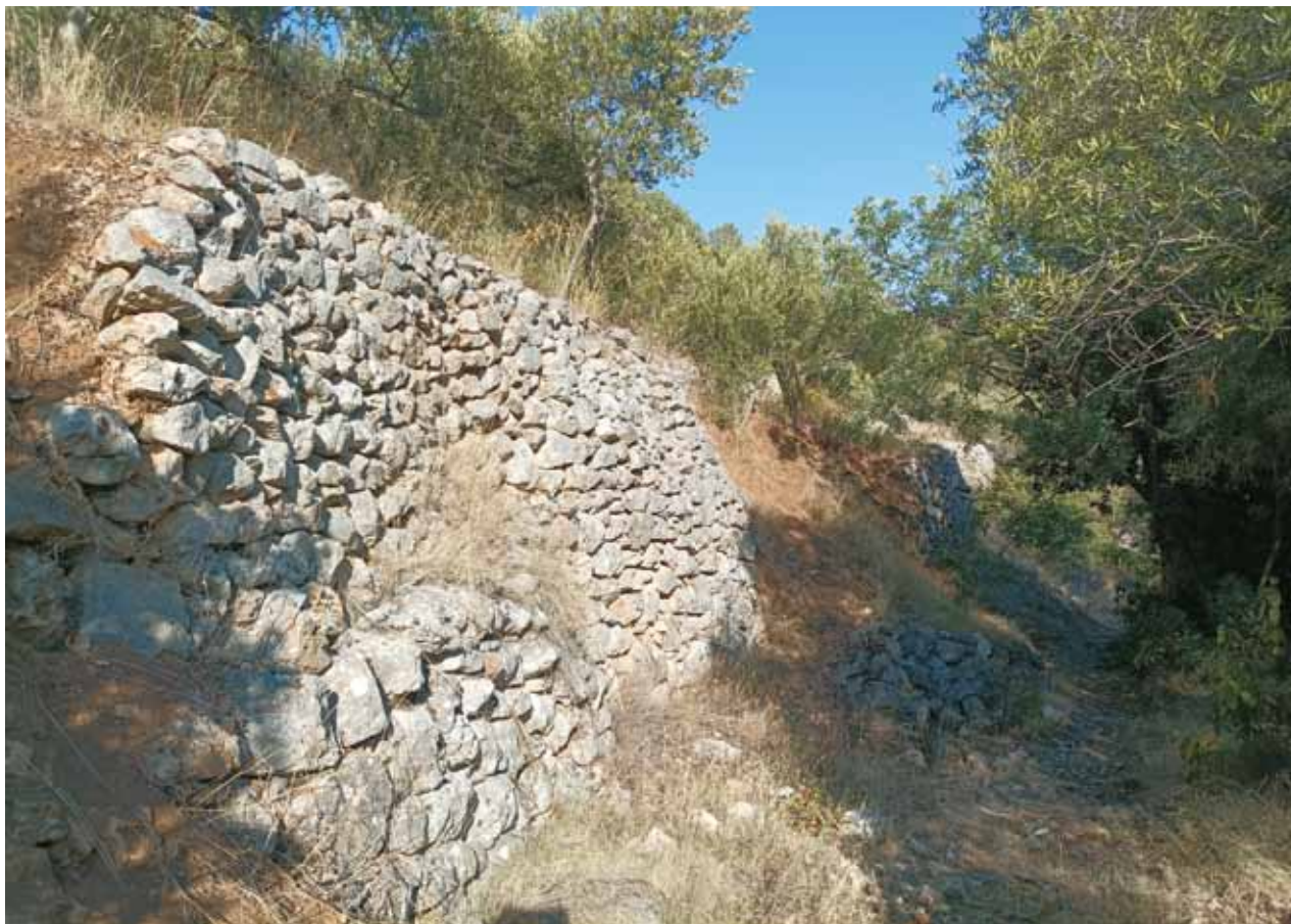
Fig. 32 – Tall dry stone wall (c. 3 m) along the paved path at the position of Laze (photo: B. Kirigin)
