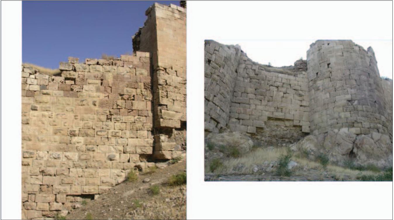
Fig. 13 Photograph of the walls showing the building style (photo by: E. Eser, 2016)
