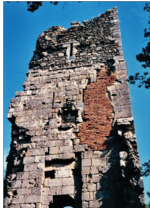
Fig. 15 Bedemgrad castle, arrow slits, the view from the outside (photo by: R. Ivanušec)
