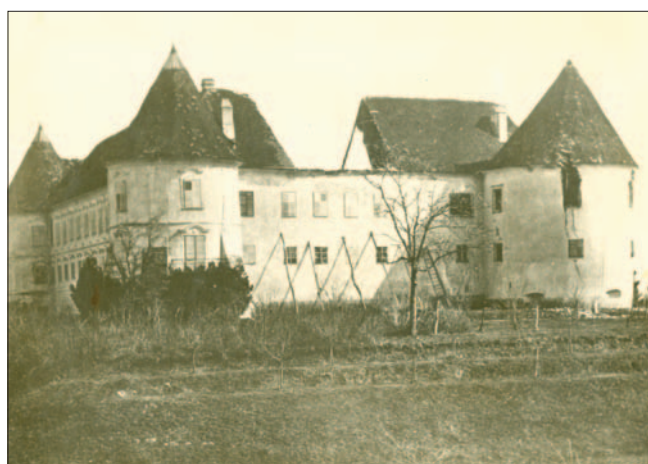
Fig. 9 Kerestinec mansion, western façade (unknown author 1880, Ministry of Culture, Directorate for the Protection of Cultural Heritage, Cultural heritage Documentation department, inv. no. 8490, neg. II-15424)
