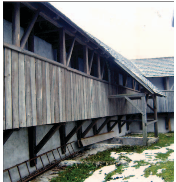
Fig. 35 Cerovo - Tabor, Slovenia: reconstruction of the wooden battlements on the walls around the parish church from 1999 (photo by: Z. Fumić)
