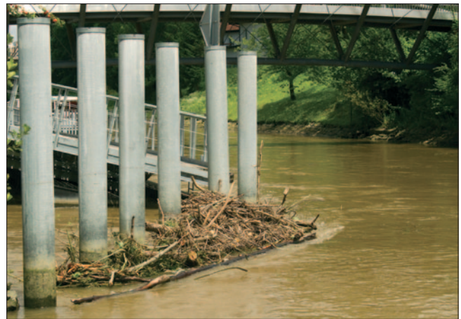
Fig. 11 The accumulation of organic material at the metallic piles of the riverine port at Špica in Ljubljana (photo: D. Valoh)
